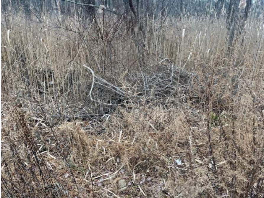
36" Diameter Pipe Outfall Covered in Brush Pile to the North of Development Area
