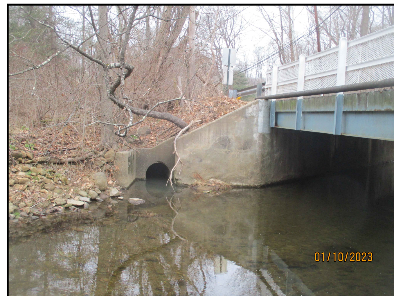
36" REINFORCED CONCRETE PIPE AND HEADWALL AT END OF NORTHWEST WINGWALL LOOKING NORTHWEST
