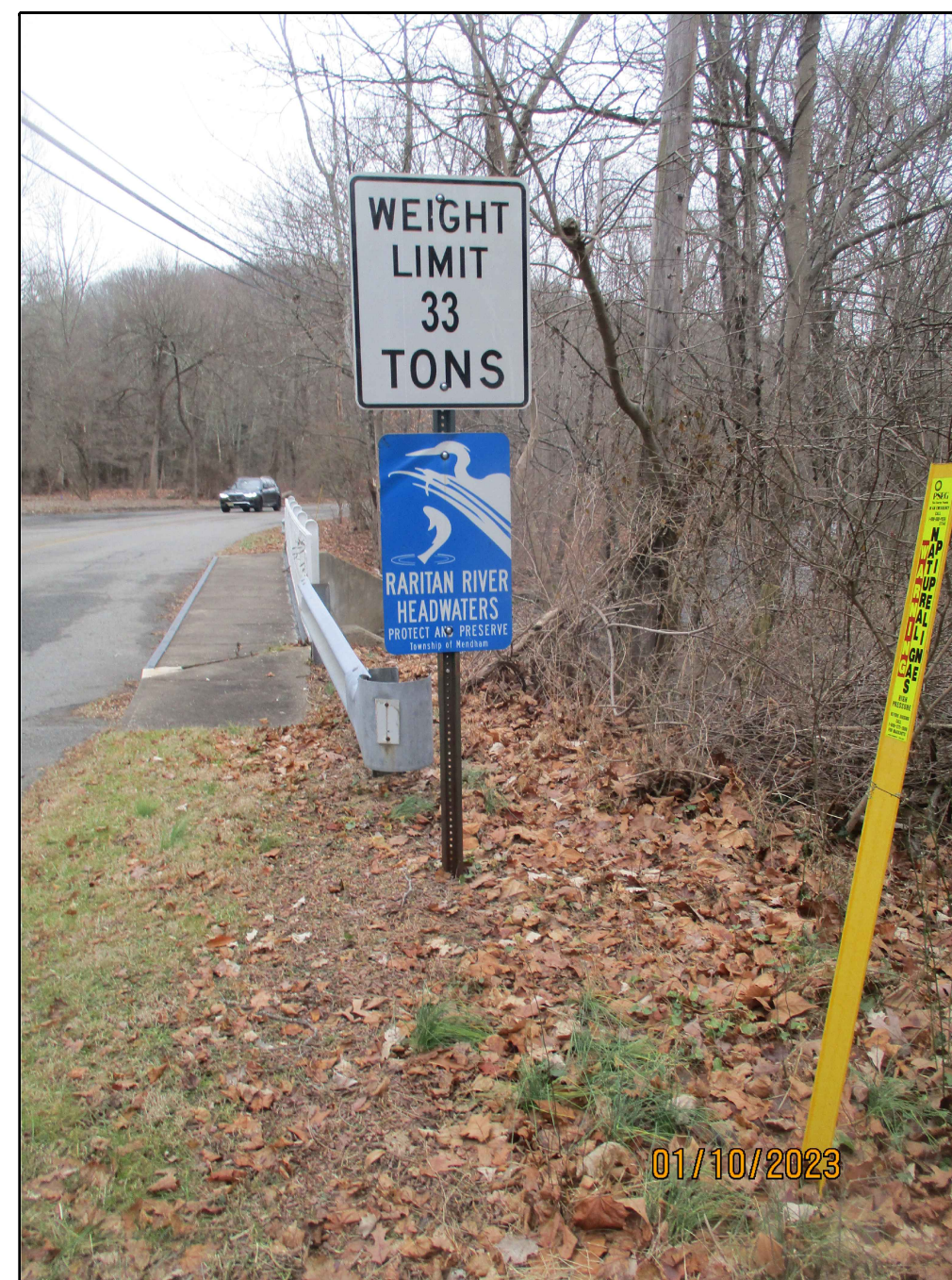
CONCRETE SIDEWALK WEIGHT LIMIT SIGN AND GAS MAIN MARKER AT WEST FASCIA LOOKING SOUTHEAST
