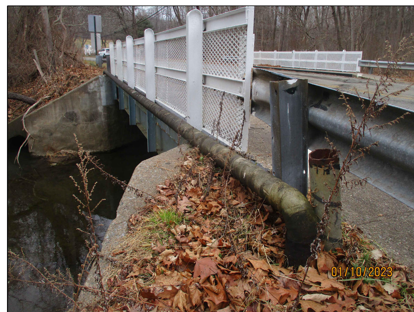
STEEL CHANNEL RAILING WITH STEEL LATTICE FACING BRIDGE MOUNTED GAS MAIN AT WEST FASCIA (DOWNSTREAM) LOOKING NORTHEAST
